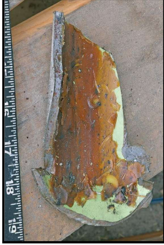
Figure 46. Detailed view of Upper Drag Strut- Inner surface. Note: Corrosion inhibiting compound (CIC).
