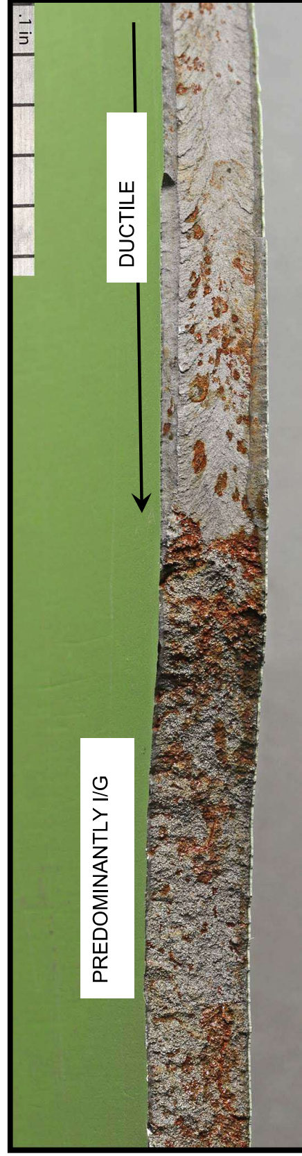
Figure 63. Detailed view of Upper Drag Strut- Longitudinal Fracture B.
